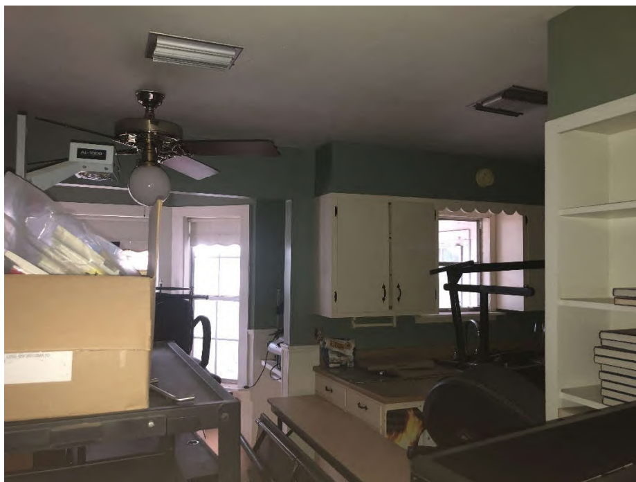
PHOTO 6: Shows the sheetrock wall system with bumpy texture sampled in the conference room, northeast office, and kitchen (Samples 13-15). Testing of this material indicated the presence of chrysotile asbestos in the wall texture and joint compound at a concentration of two (2) percent.
