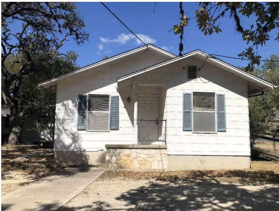
PHOTO 9: Shows the exterior siding (Samples 22-24) with black tar paper behind it (Samples 25-27) sampled from the exterior of the structure. Testing of the exterior siding indicated the presence of chrysotile asbestos at a concentration of thirty (30) percent. No asbestos was detected in the exterior tar paper behind the siding.
