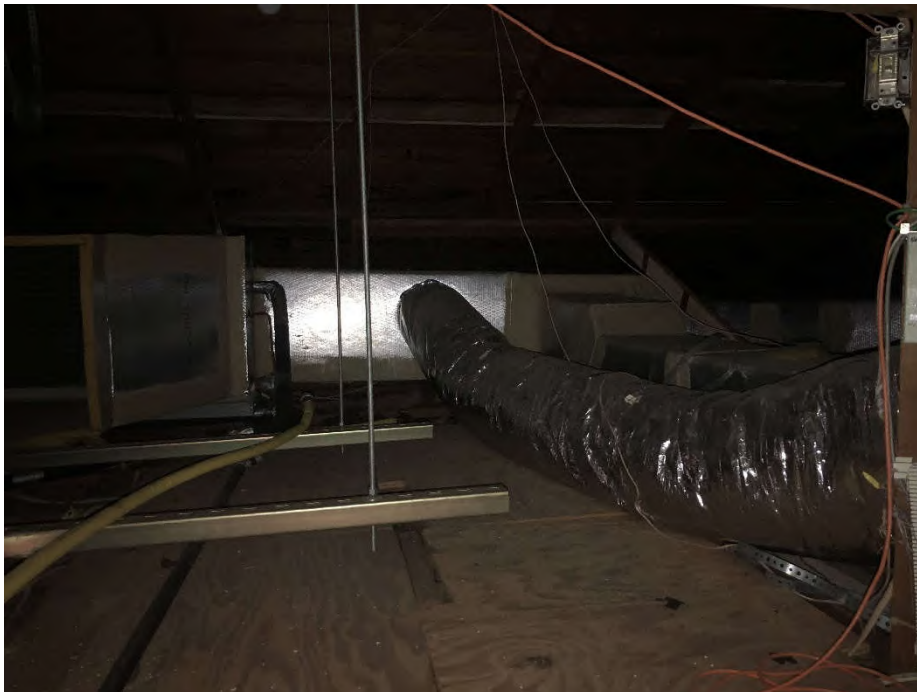
PHOTO 8: Shows the off-white mastic on HVAC ductwork sampled in the attic (Samples 19-21). Testing of this material did not indicate the presence of asbestos.
